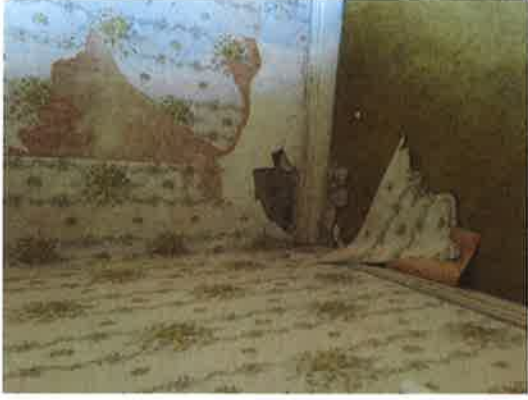
28. Damage to plaster
